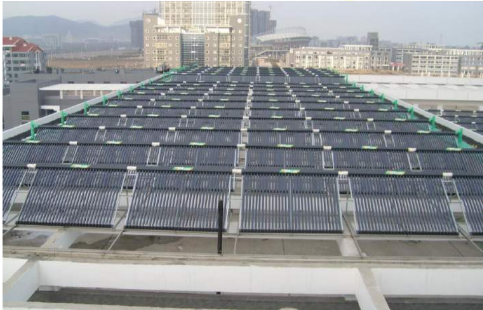
Solar hot water project for Binzhou medical university
