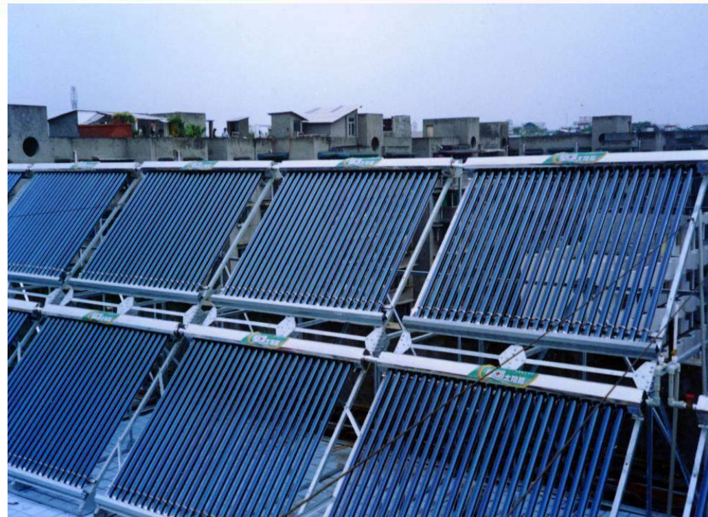
Solar hot water project for Meishan middle school, Sichuan province
