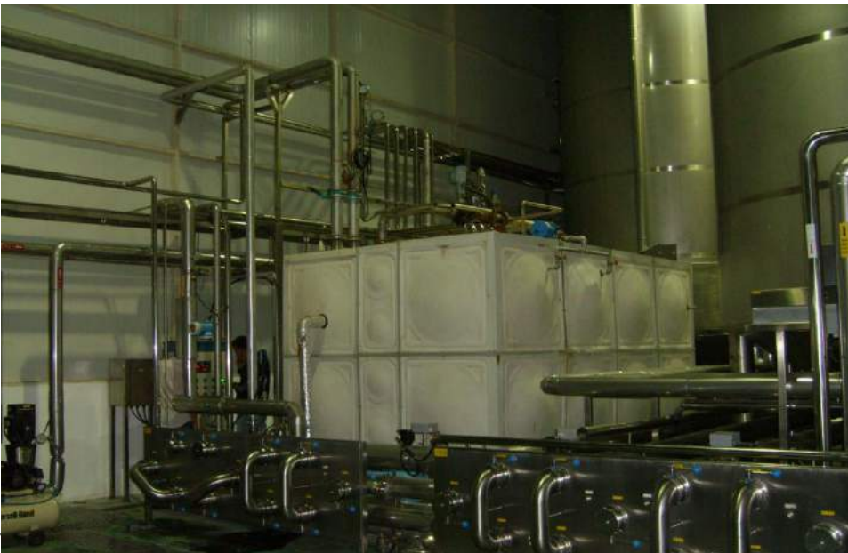
← Water tank room of Pepsi~Cola Harbin factory solar hot water project
