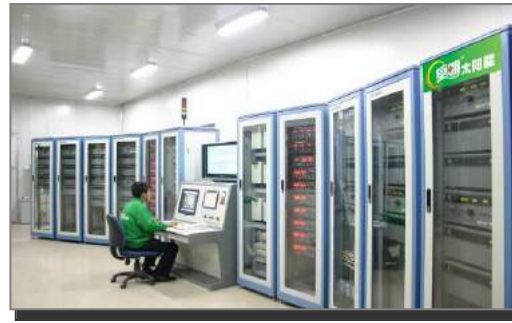
Vacuum tube coating control center
