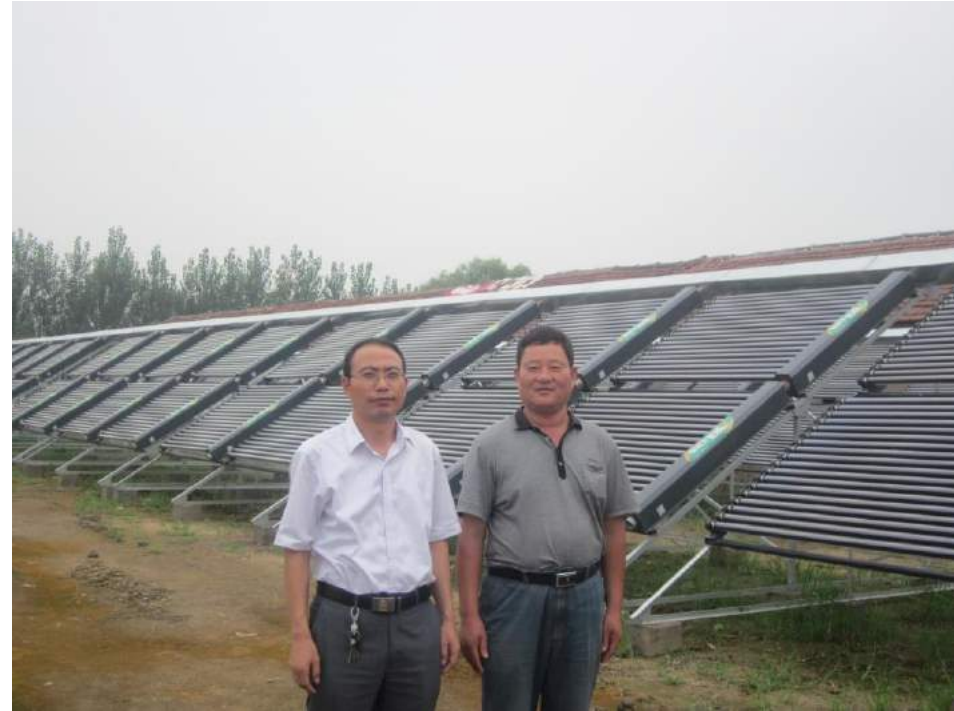
Solar drying project for Sludge disposal project of Jinan Government
