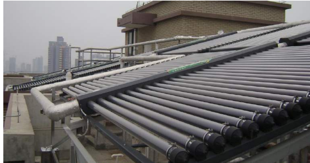
Solar hot water project for Licai yihe real estate project, Xianyang city
