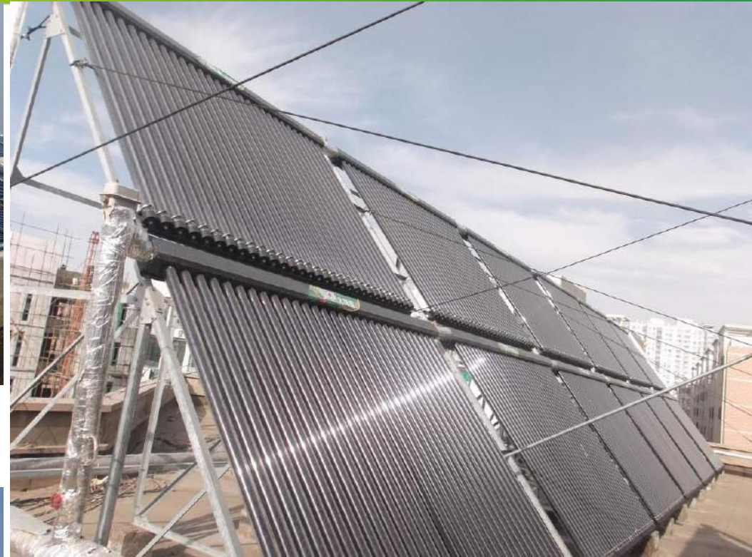
Solar hot water project for Bazhou Special-education schools, Xinjiang
