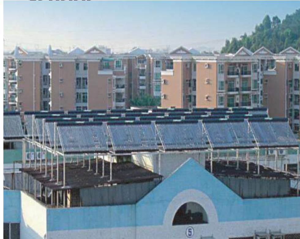
Solar hot water project for Biguiyuan school in Guangdong
